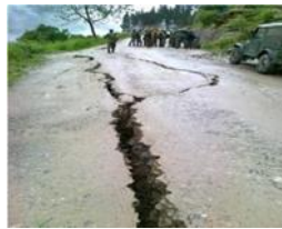
Fig 10: Earthquake damage to roads
